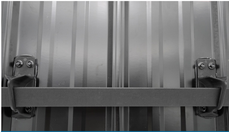
Figure 6 — Rail seated in the brackets. The rail runs continuously through the slot in each upright, carried above the panel across the whole run.
